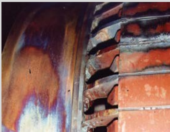
Rotor core damage due to broken bars
